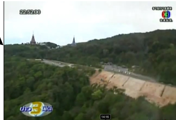
Localised slope failure (highway slope)
